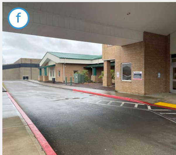
Angled crosswalks diverge at the singular curb ramp at the front entrance to walkways in the parking lot, creating long crossing distances.
